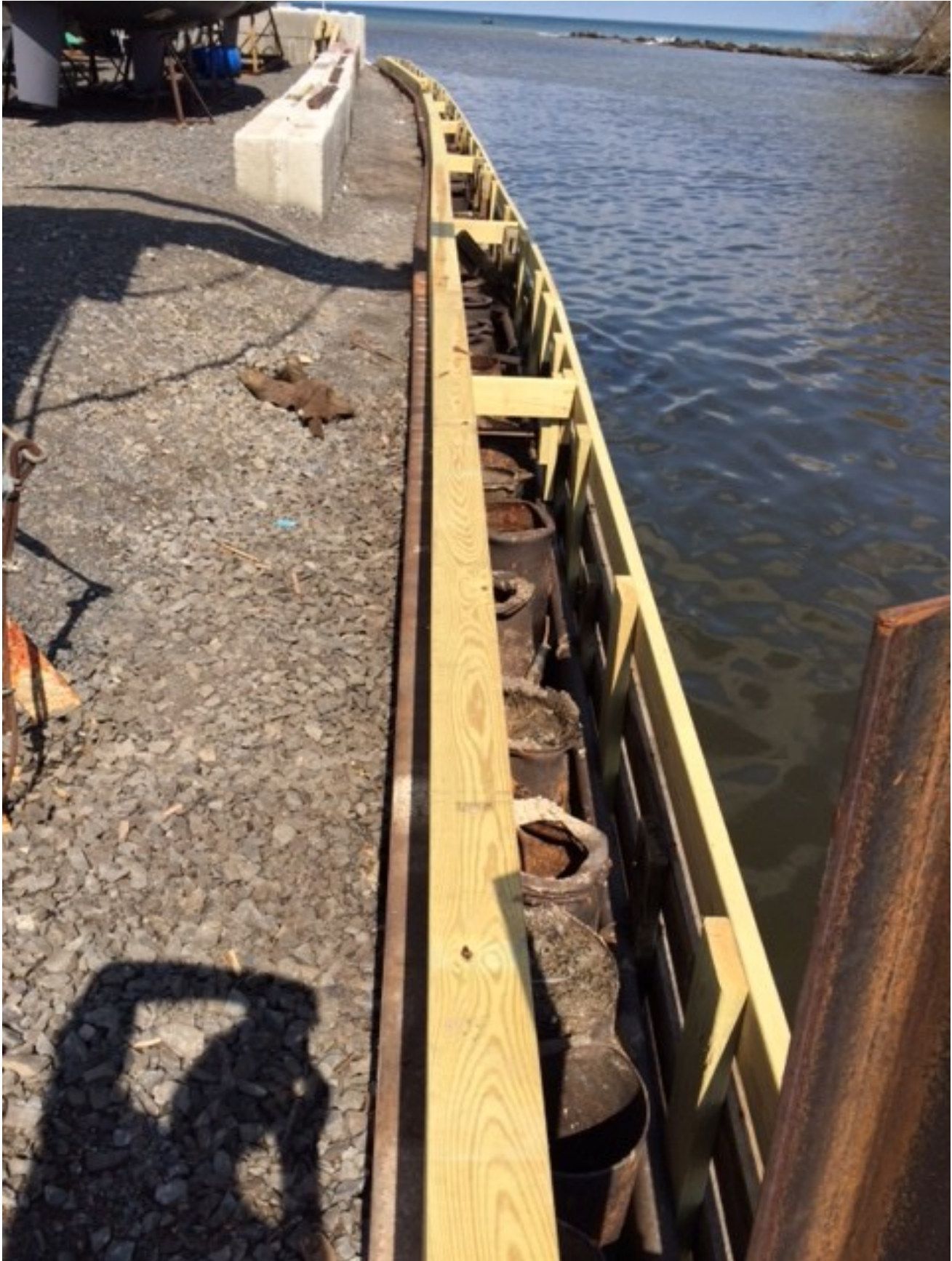
Seawall Visitor Dock Progress. Great work by Dave Manning and his crew.
