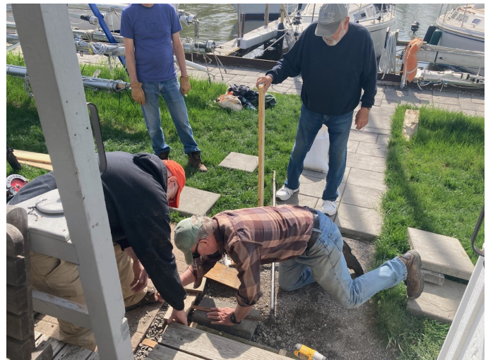
Paul Ward and crew building a safe steps and railing at the club opening.
