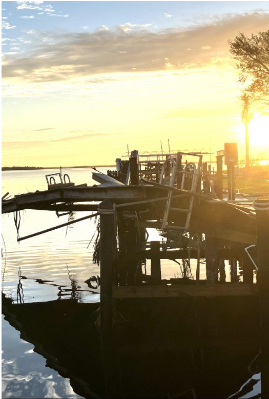
Sept 29 2022. After Hurricane Ian Fort Myers Beach. Dock damage.
