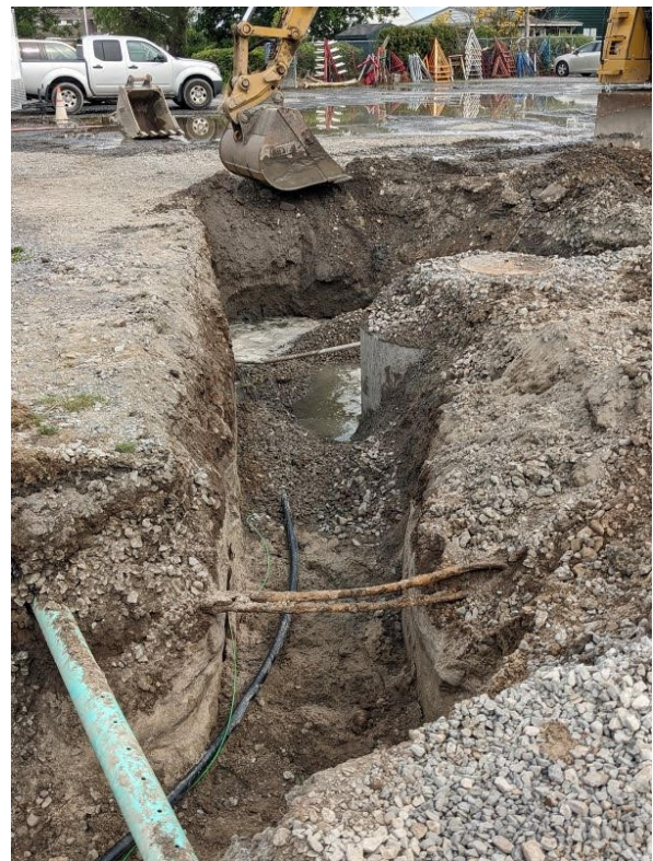
Looking W-NW: Existing perforated drain pipe, elect. conduits, mystery water line, & concrete end-of-line manhole.
