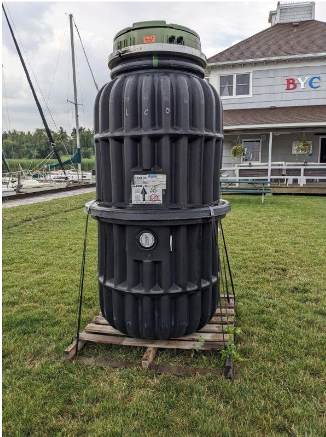
Pump(s) prior to installation.
