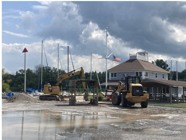
The construction team puts in the final pieces of the sewer at the club. Photo credit: Rich Wiest
